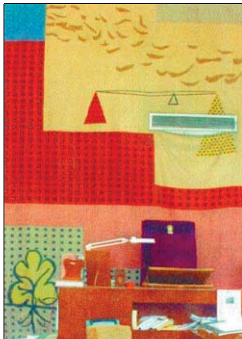
Detail of tapestry in Court 6: The 'counterbalance of complexities' and the 'tree as a symbol of perfection'. Air-conditioning ducts puncture the tapestry indiscriminately, mutilating motifs.
